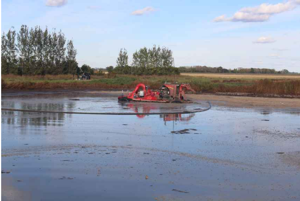
Nuhn boat agitator/pump feeding drag hose applicator in primary cell at first strategy
